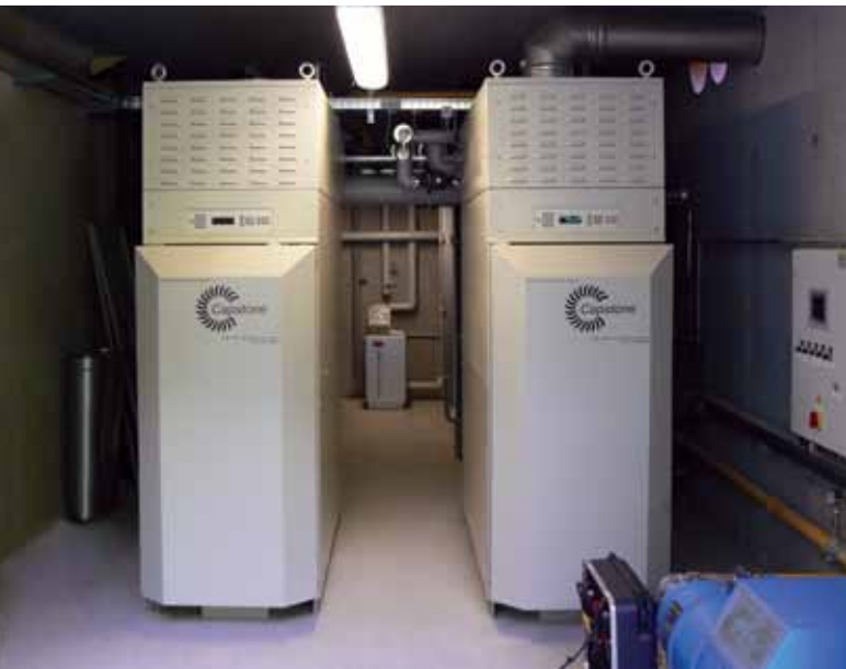
The cogeneration system generates 1 million kWh of electricity and 1.8 million kWh of thermal power onsite, exceeding 80 percent energy efficiency.
