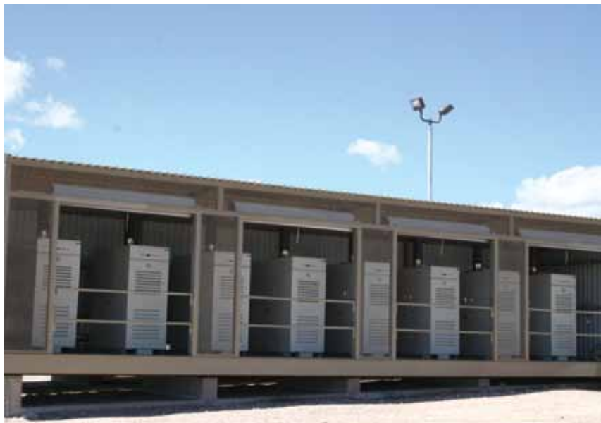
Fifteen 65kW microturbines provide the primary power for this oil pipeline booster station in New Mexico.
