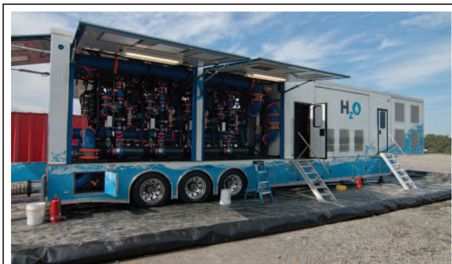
Hydrozonix LLC is expanding its fleet of EF80™ treatment units to service fracturing operations in the Permian Basin and the Marcellus Shale, with the company planning to build two units each quarter over the next two years, depending on market demand. Each EF80 unit can treat 80 bbl/minute during fracturing and post-frac flow back. The systems use the patented Ozonix™ oxidation process that incorporates ozone, hydrodynamic cavitation, acoustic cavitation, and electro-chemistry for microbial control and scale inhibition.
