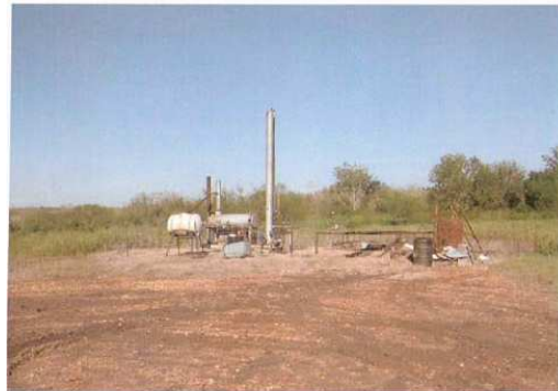
Photo No. 3 – Patrick Welder Tank Battery
