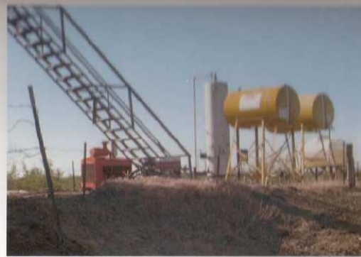
Photo No. 2 – Patrick Welder Tank Battery
